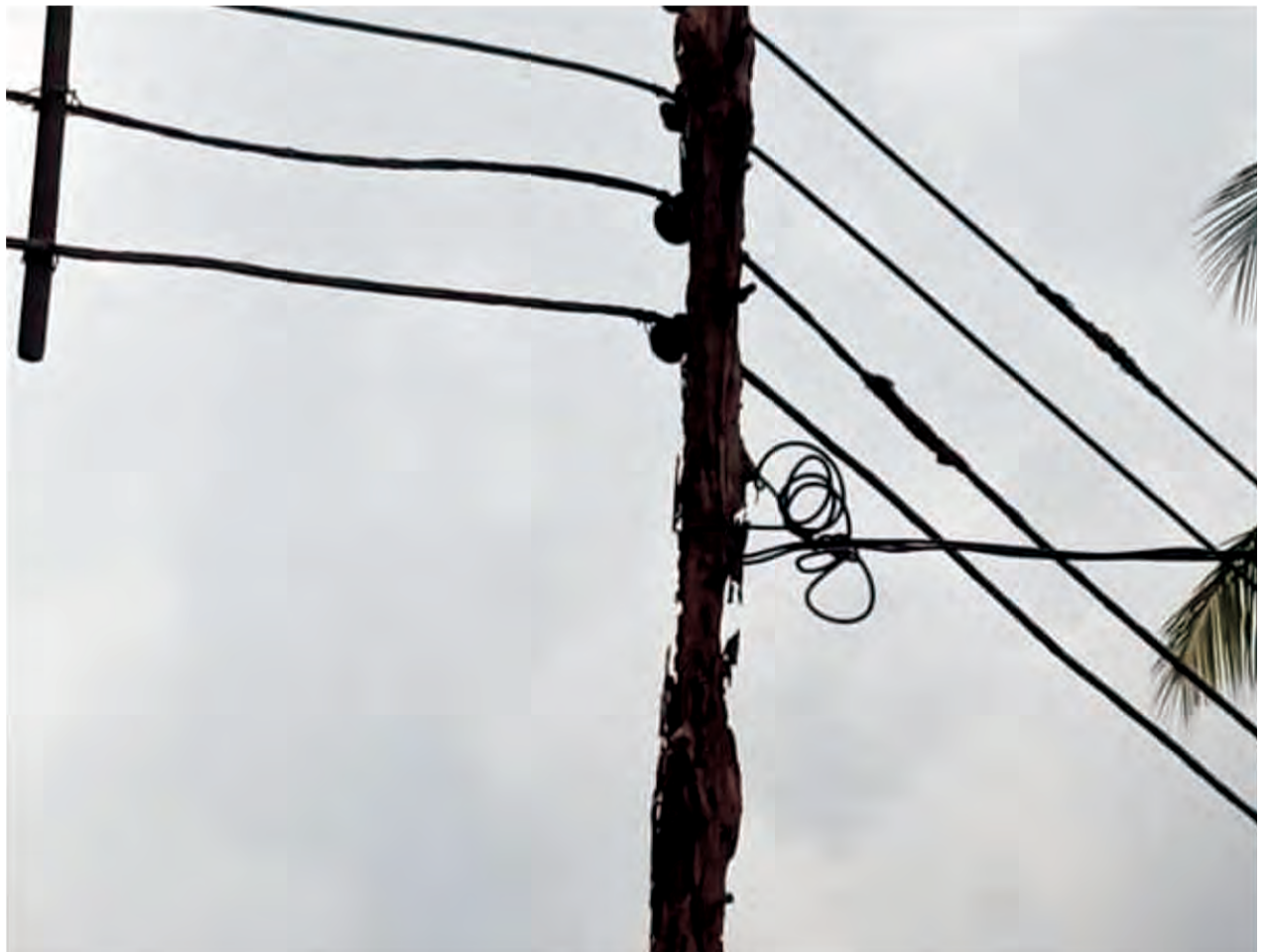
Termite eaten electricity pole at Sanusi street
