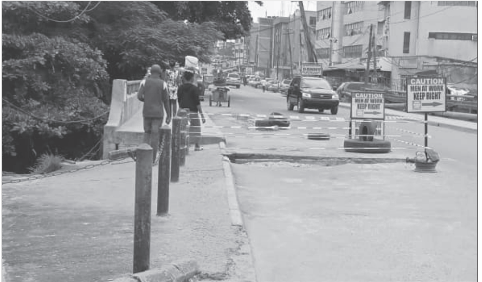
The failed portion of Osolo Way
