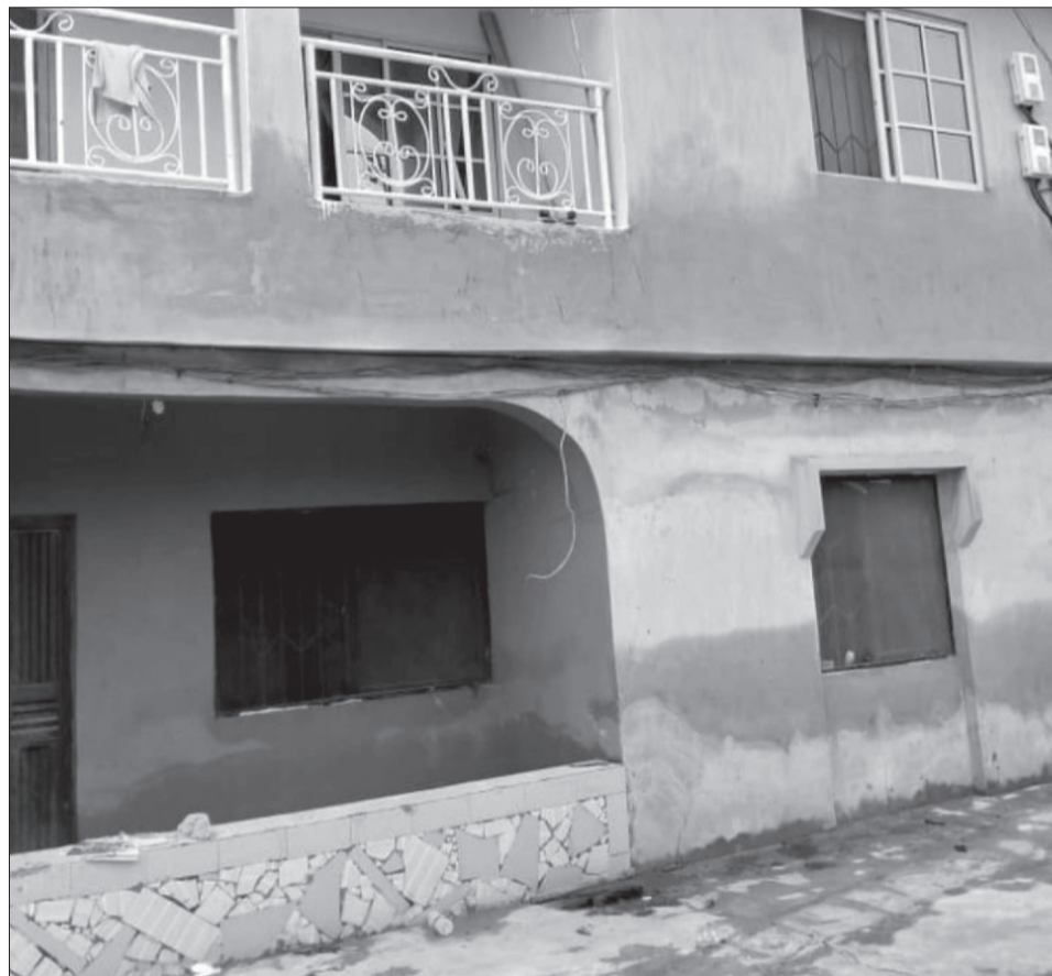
The house which always get flooded to send tenants packing during rainy season, at sewage area, Jakande Estate Ejigbo
