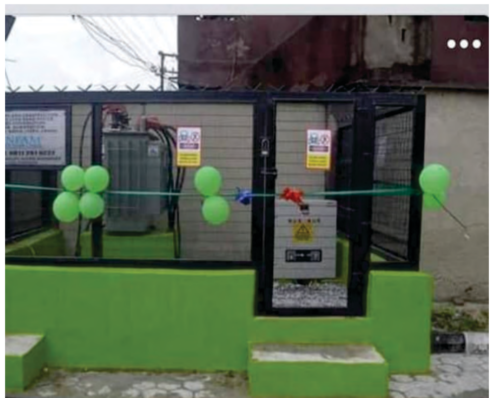
The new installed transformer
